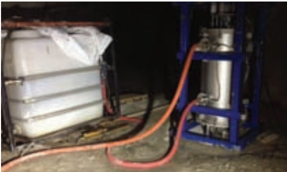
Above, left to right: the filtering system from Ramson; the water-propelled drilling equipment in use
